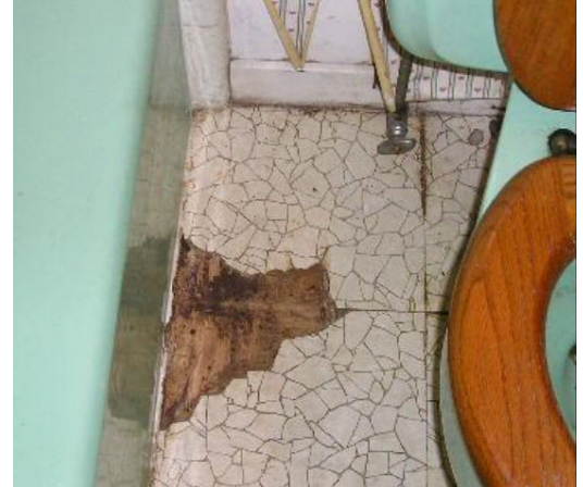
Bathroom floor damage
